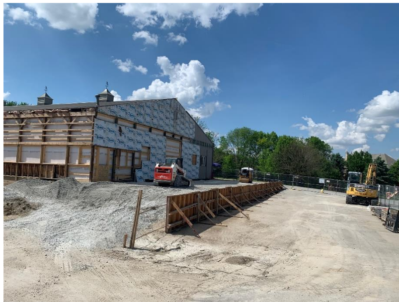
The new office space will come out thirty feet to the east side of the building, and will house our admin team.
